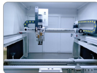
Coating system chambers
